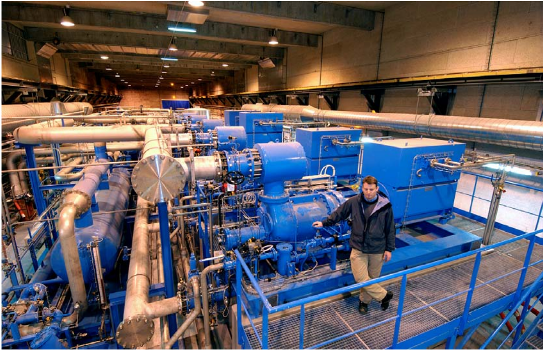
a) Compressor station
